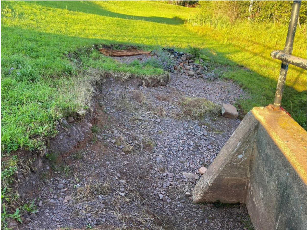
FIGURE 11. AREA OF INTEREST ON THE LEFT EMBANKMENT (WEST WINGWALL) FACING DOWNSTREAM AT THE TOW OF THE EMBANKMENT (August 30, 2022).
